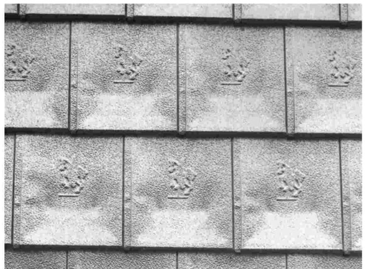
Close-up of the copper shingles used in the carousel's fascia reveals an embossed design mirroring the copper horse atop its copper-shingled roof.
