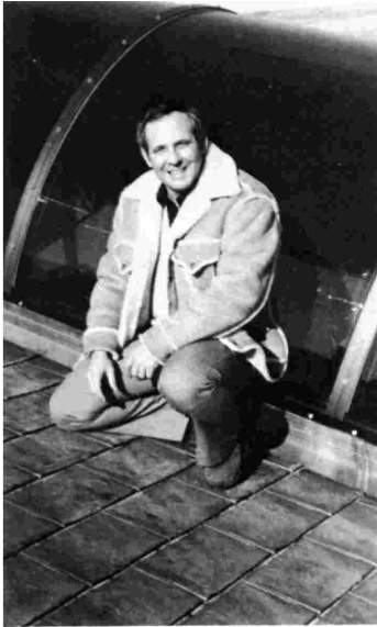
Seen on a new copper shingle roof is manufacturer Joe Zappone, who says that because of the installation speed possible with his copper shingles, the home owner is putting his money into product quality rather than labor.
